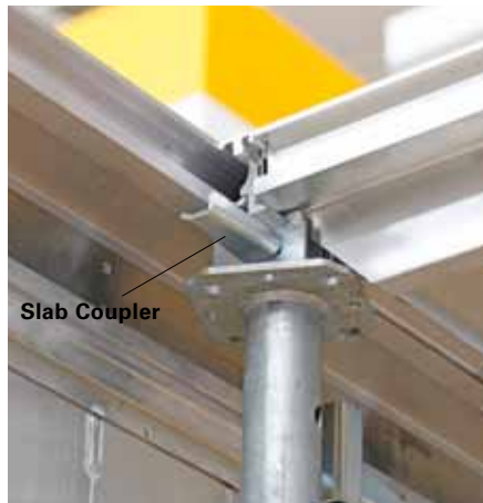
Connect the Slab Beam and Transition Panel with Slab Couplers and support with slab props.
