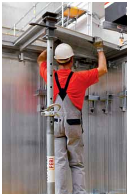
Insert the first Slab Panel and secure on three sides with Slab Couplers.
