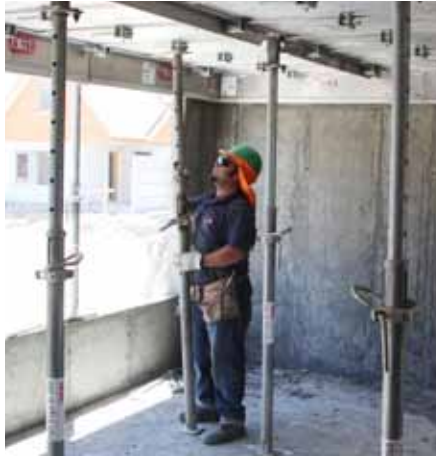
Position the temporary support before striking takes place. One temporary support per 5 Slab Panels, left and right.
