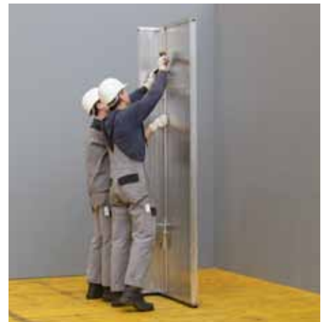
Connect the Wall Panel and Corner Panel with Wall Couplers - see plan for number of couplers used.
