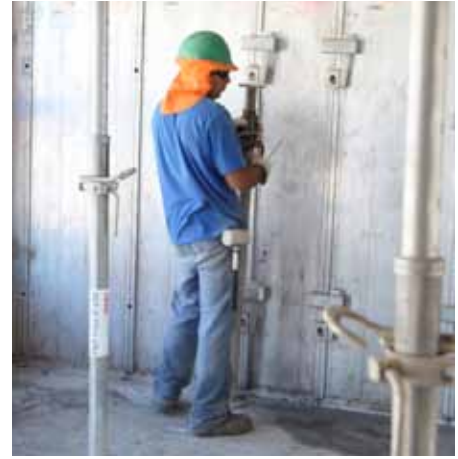
If necessary, remove slab props from the Slab Beam-Transition Panel transition area.
