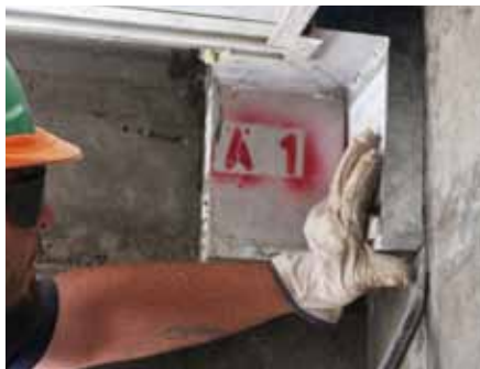
Release Transition Corner from the concrete.
