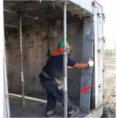
Dismantle the Stop End Profiles - remove from concrete from bottom to top.
