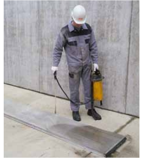
Apply release agent before positioning the panels, also on the front sides.
