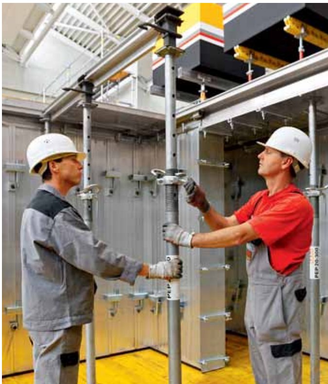
Position slab prop in a vertical position and carry out any necessary height adjustments.
